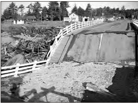
Figure 3. Damage to the State Highway 109 bridge over the Copalis River near Copalis Beach caused by a distant tsunami from the 1964 Alaska earthquake. Courtesy of the Daily World , Aberdeen, Wash.
